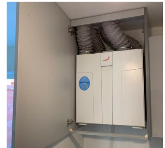
Fig 68: Example MVHR installation (credit: Zehnder)
